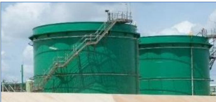
Photograph 2-2: Oil will be stored in 10,000 m 3 tanks with floating roofs. Temperature in the tanks will be maintained at 68°C.
