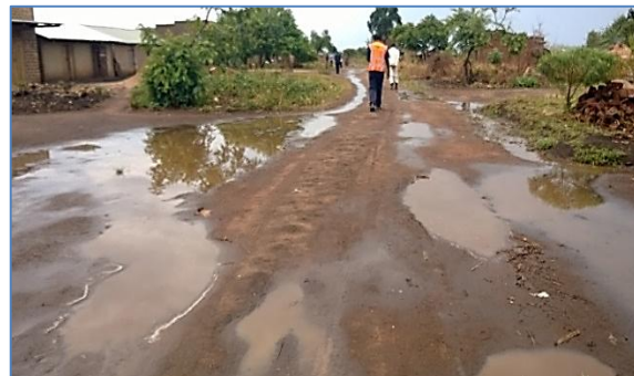
Photograph 6-30: As elsewhere in the District, local roads along the pipeline route are in need of repair
