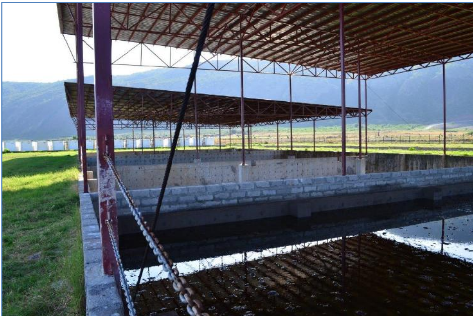
Photograph 8-1: Current arrangements for the temporary storage of drilling waste on the Buhuka Flats
