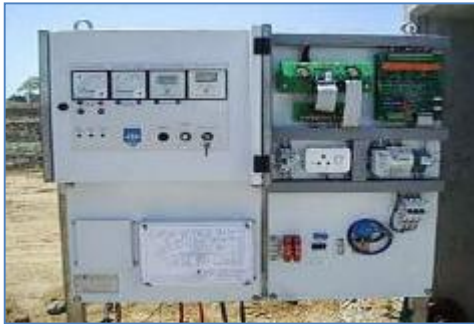
Photograph 2-2: CP instrumentation. The instruments provide information to maintenance teams which demonstrate that the cathodic protection is working properly.
