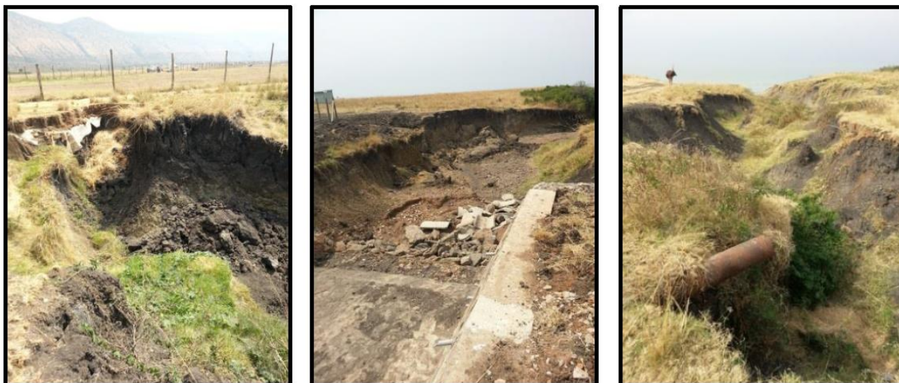
Figure 13: Evidence of soil erosion at the Kingfisher Field Development Area
