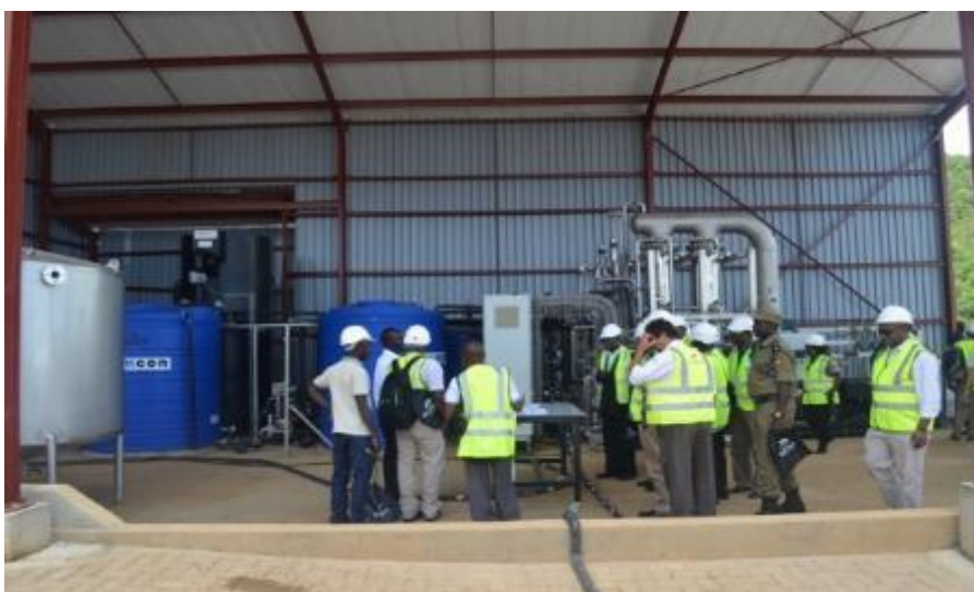
Figure 10: Leachate Treatment Plant at EnviroServ
