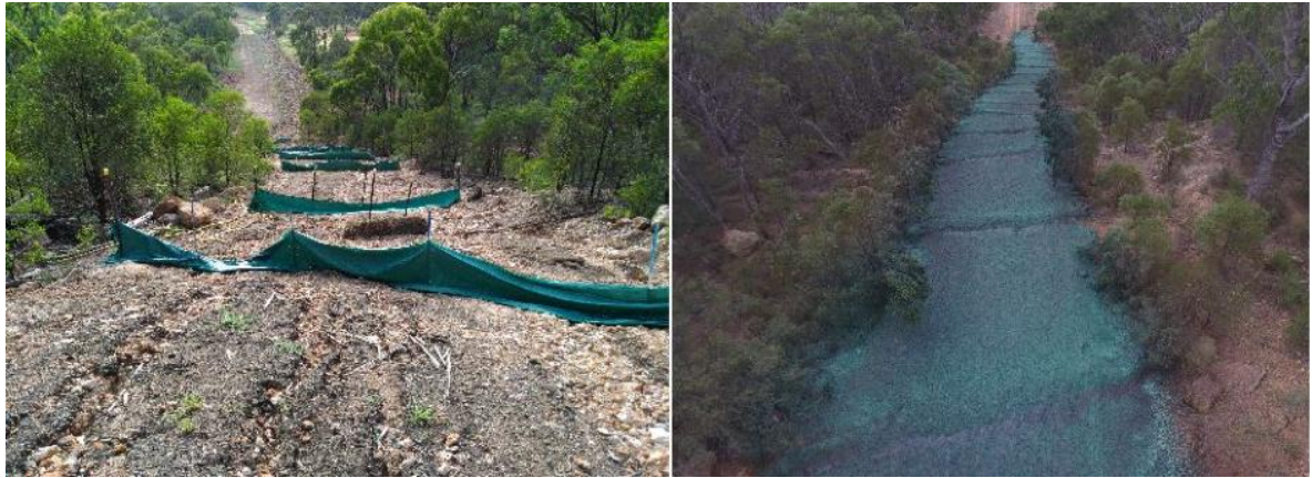
Initial backfilled pipeline corridor along a steep embankment protected against erosion with mulch and sediment netting (left) and subsequently soil binding polymers (right)
