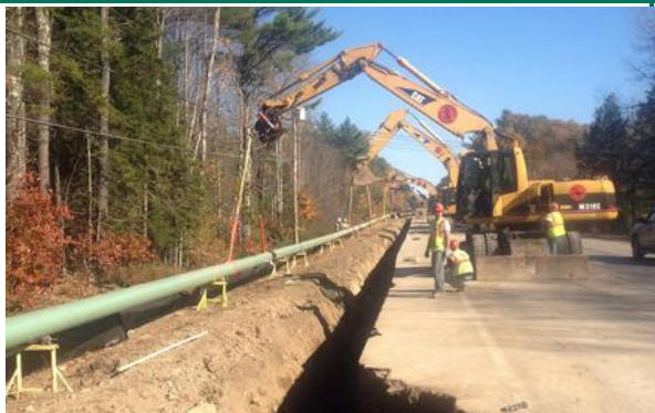
Positioning of a pipeline within a servitude using an existing road as access way
