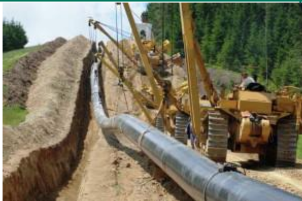
Positioning and lowering of a pipeline along an existing servitude/clearing through a wooded area
