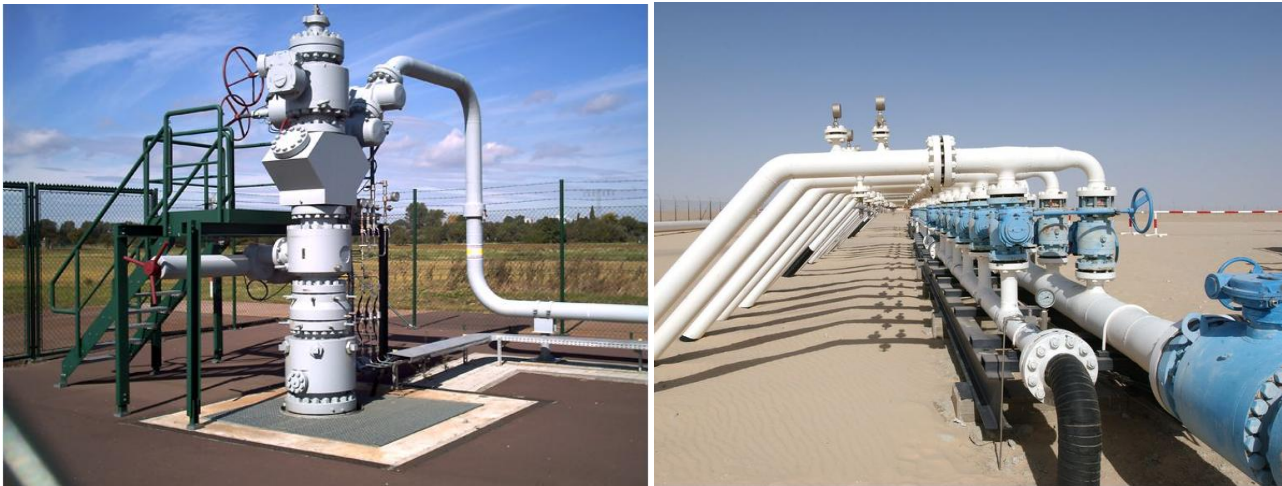
Figure 28: A well head (left) and production manifold (right) (for illustration).
