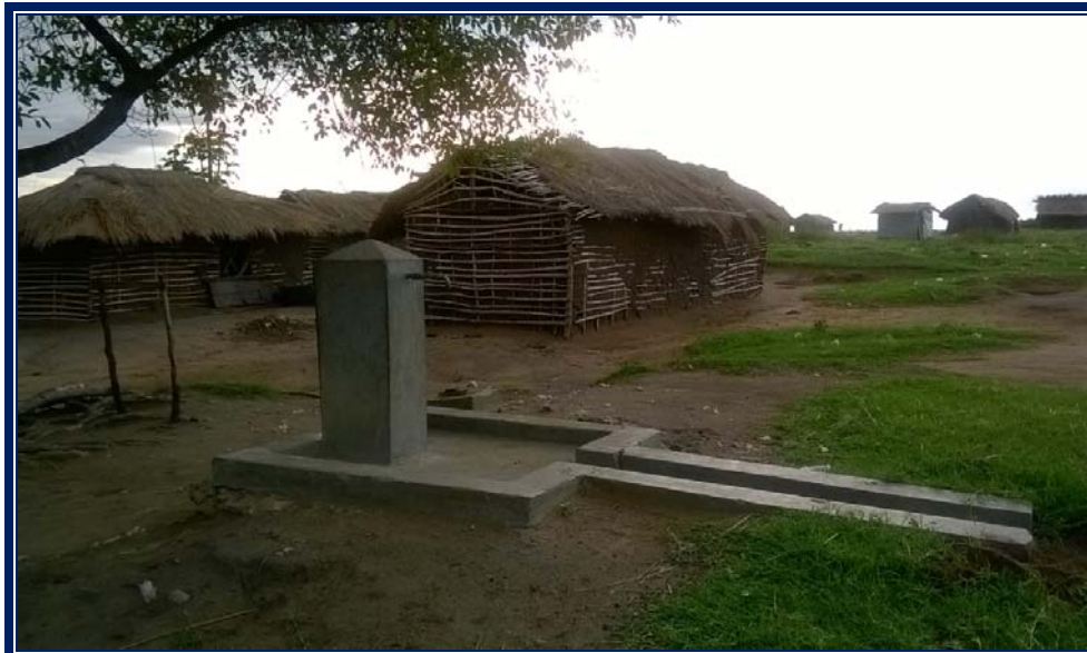
Figure 25: Non functional tap from gravity fed water scheme in Kacunde
