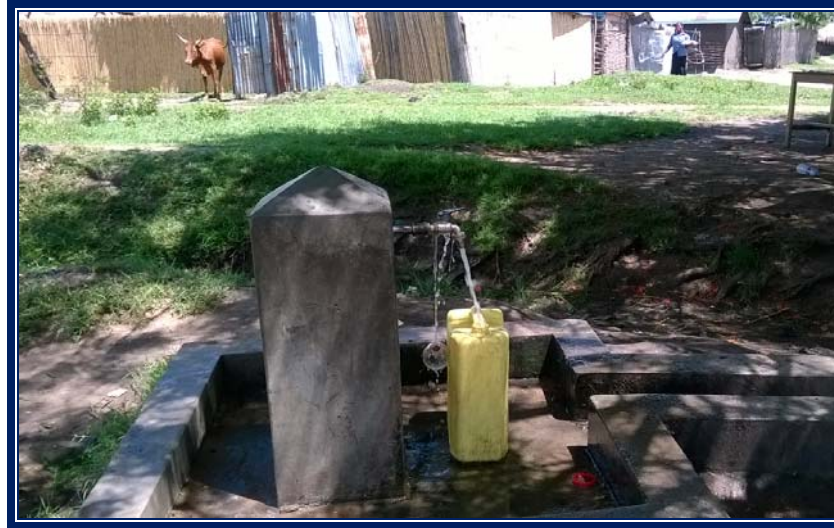
Figure 26: Functional gravity fed water tap in Nsonga
