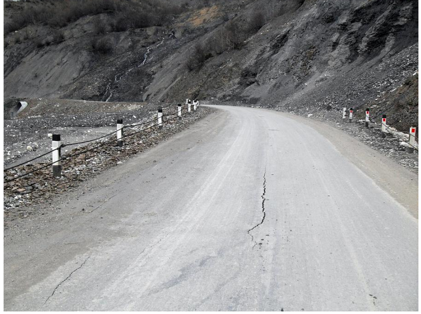
Photo 19. In sufficient road drainage cause instability in the road foundation and leads to landslides.
